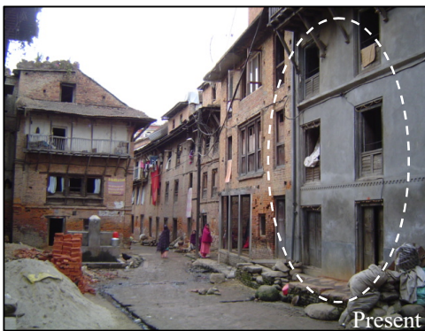
Fig 8 (b) Change of mud brick façade building to cement plastered (dotted part in Fig 8 (a))
